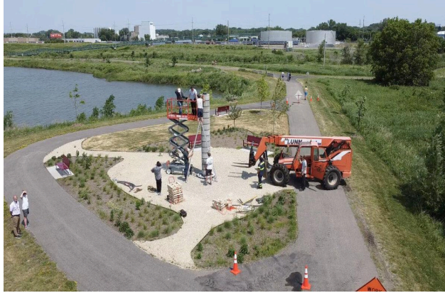
Installation of Pillar Sundial by C. Anthony Huber, Cascade Lake Regional Park, 2021.
